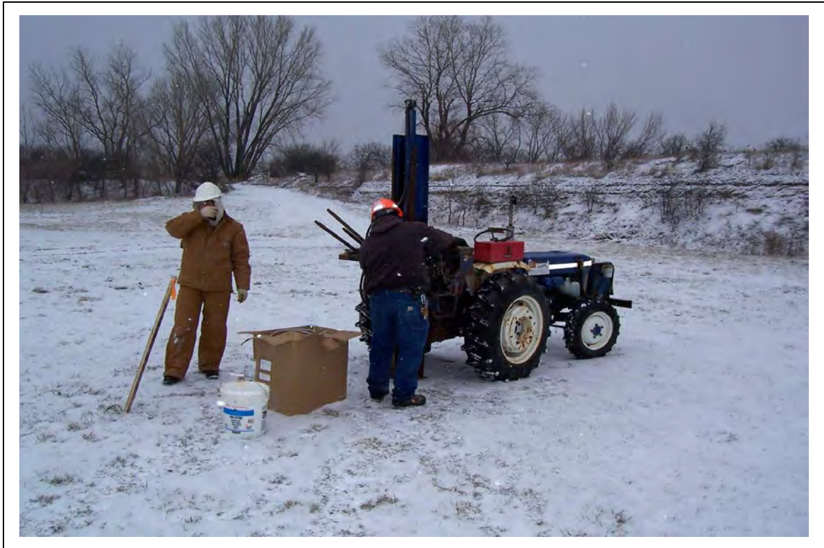
Photo 13 – View of VI-03 installation
